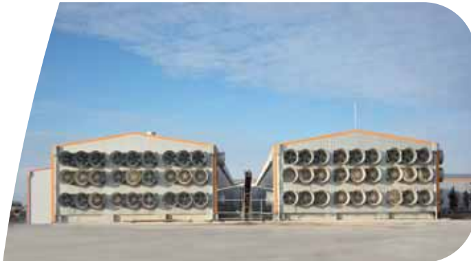
Coop ventilation outlets
